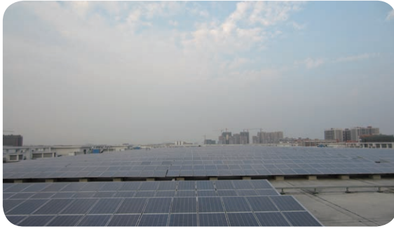
Huawei solar power station
